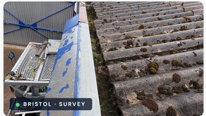
Same survey, at the eaves: biological growth concentrated along gutter lines and fixing rows — exactly where Hipolava dwell time and fastener remediation earn their keep.
