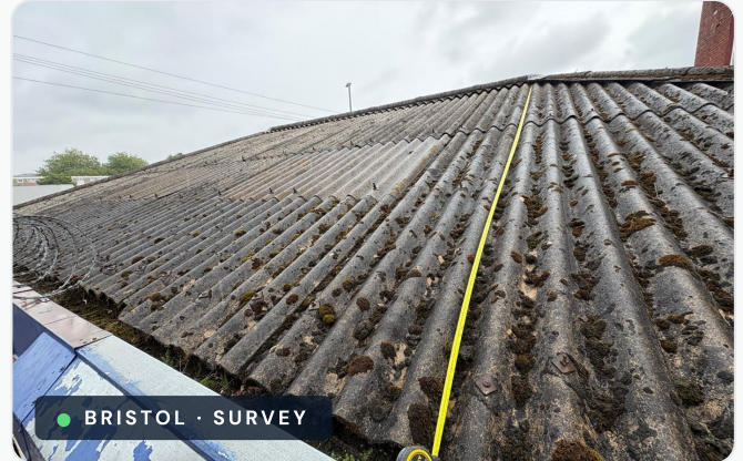
Survey photo, Bristol: an aged asbestos cement roof with heavy moss growth and corroded fixings — specified for a foam + U91/U92 overcoat system. This is the condition preparation has to reverse before any coating goes down.
