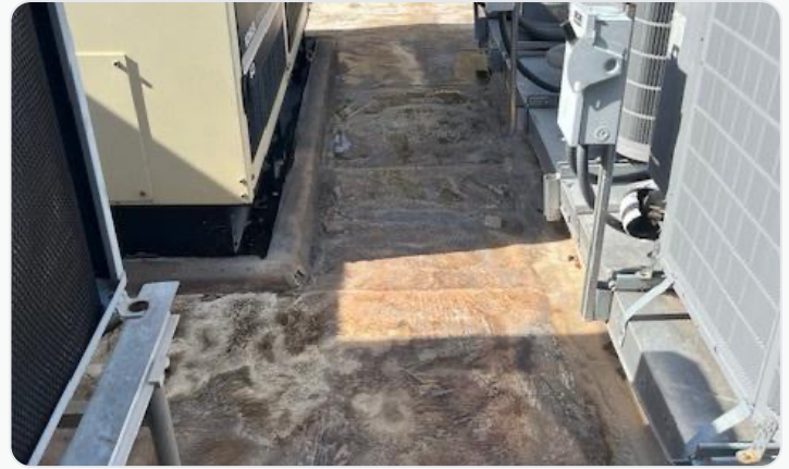
Fig 1. Oil & tar bleed-through where no Bleed Trap primer was used over aged asphalt — extreme reaction in hot weather. A clear case for specifying A4271 as a belt-and-braces measure.
